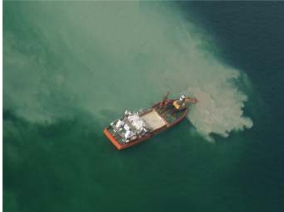
Figure 9.36 Example of sediment plume resulting from dredging works during the construction works of the offshore wind farm Nysted II. Photo: Martin Laczny.
