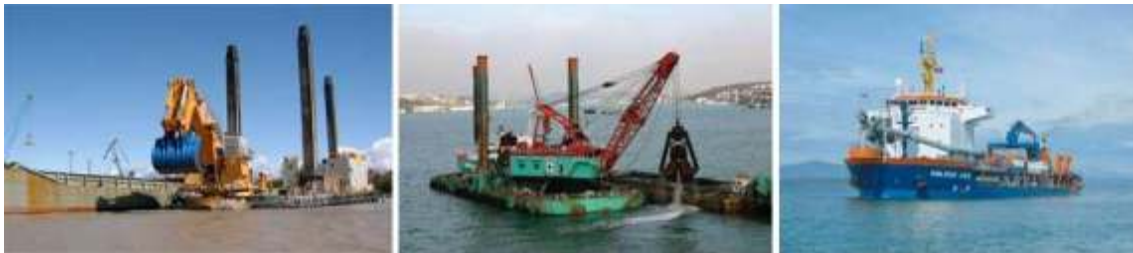
Figure 9.63 Different types of dredgers planned to be used for the construction of an immersed tunnel (from left to right: BHD "Nordic Giant" (Boskalis), GD "Kanyo" (Taisei), TSHD "Volvox Asia" (Van Oord); pictures taken from Femern A/S Consolidated Technical Report, version June-6, 2011).
